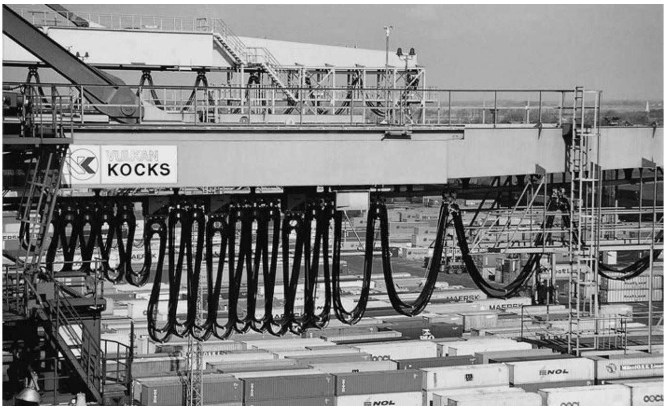
VAHLE cable carriers in Bremerhaven
